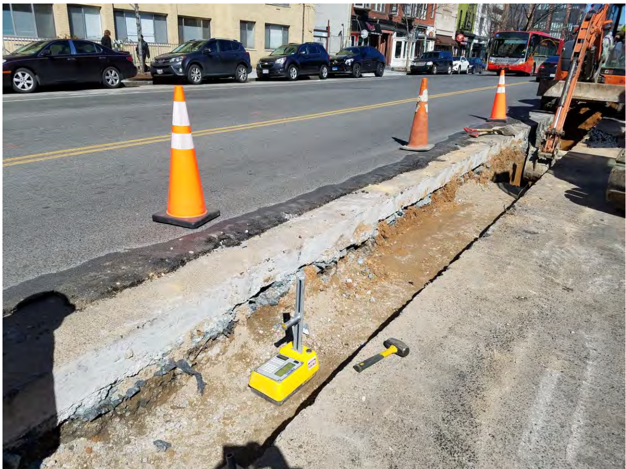
Compaction Testing between N Street and Rhode Island Ave on the Eastside
