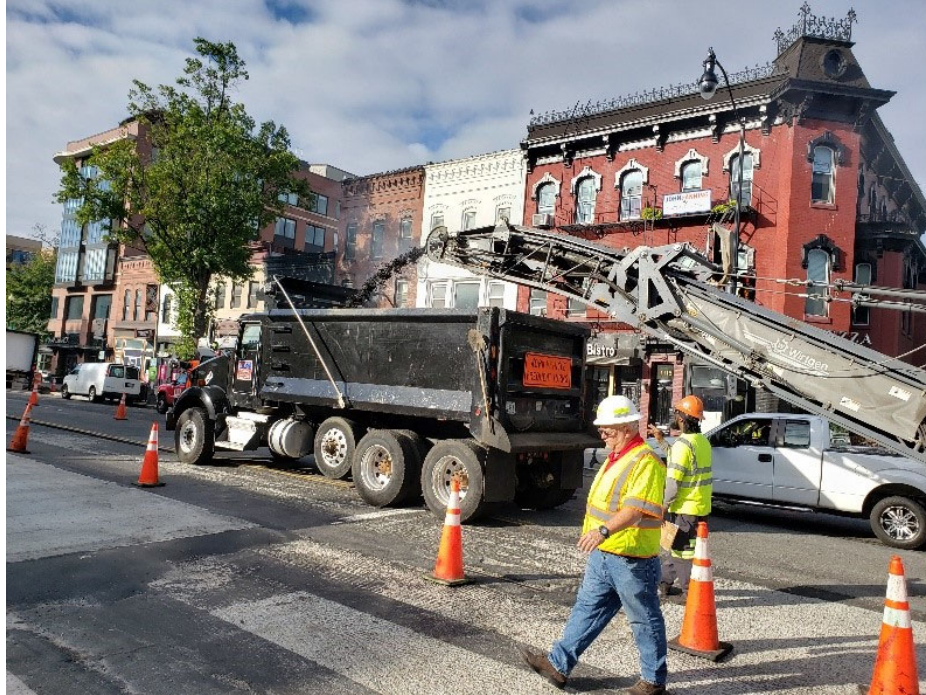
FMCC Asphalt division utilized Flaggers and Spotters plus MOT signs & Cones for Traffic Safety per DC-DoT.
