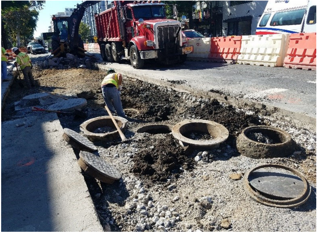
Multiple utility manholes to be adjusted and repaired.
