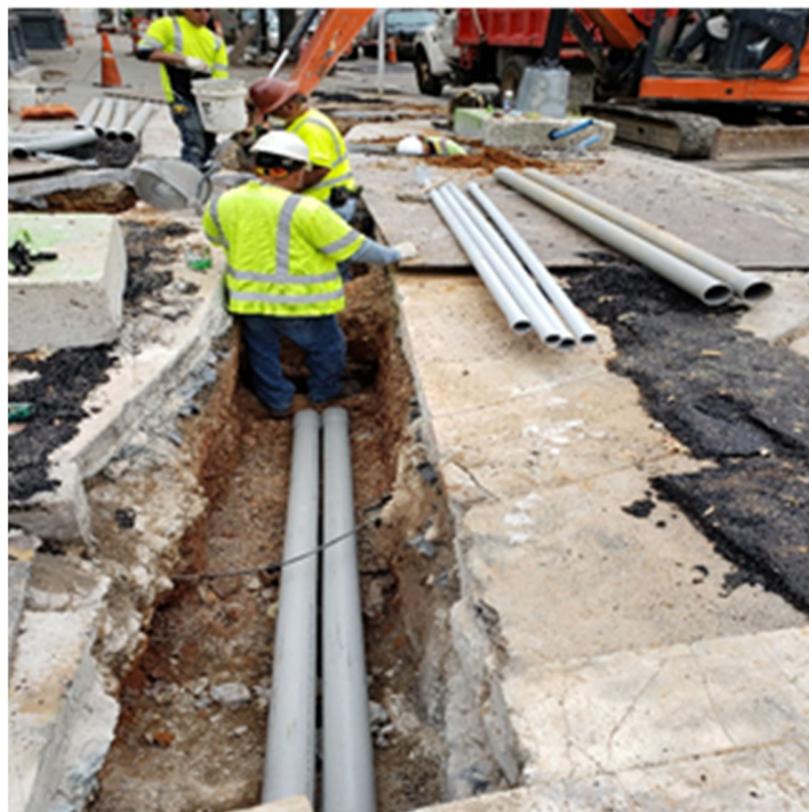
Omni, Inc. crew excavated and installed 2" & 4" Conduits for Traffic Signal Lights & then placed Class B Concrete for TS Conduits-Duct Banks, On Tues. 10-8-2019.
