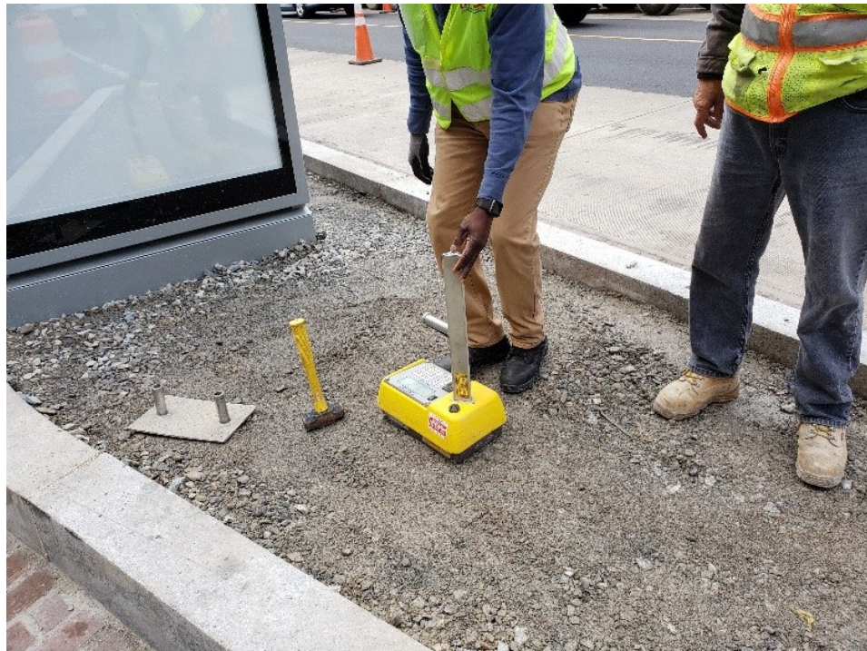
DC DoT Geotech Rep conducted several Nuke Compaction Tests for GAB Materials placed & Compacted by FMCC for Bus Island Directional, on Wed. 10-9-2019.
