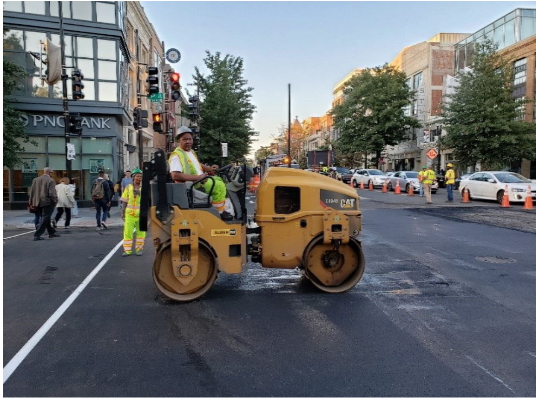
FMCC Asphalt Plant No. 2 Broke down which caused delay and switch to Plant No. 1 in Asphalt delivery and paving operation to finish at 7:45 P.M. on Friday, 10-11-2019.
