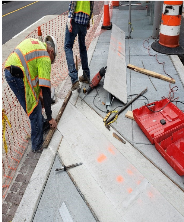
FMCC crew installed Steel Frames and Crates for Storm Channels at Bus Island at R.Island Ave. & 14th St. NW in front of 7-11 Store
