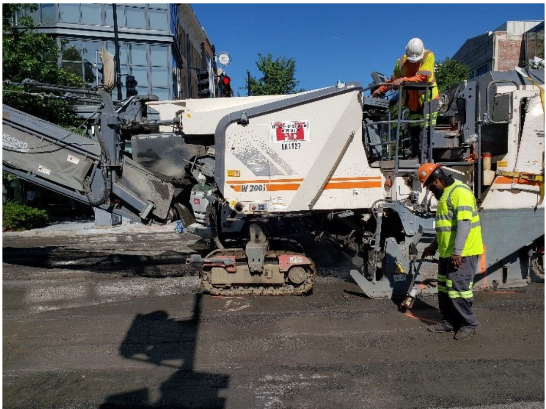
FMCC utilized MOT arrow boards, Orange Barrels and Cones to manage and maintain safe and efficient Peds, Bike and Vehicle traffic during the evening and night Milling
