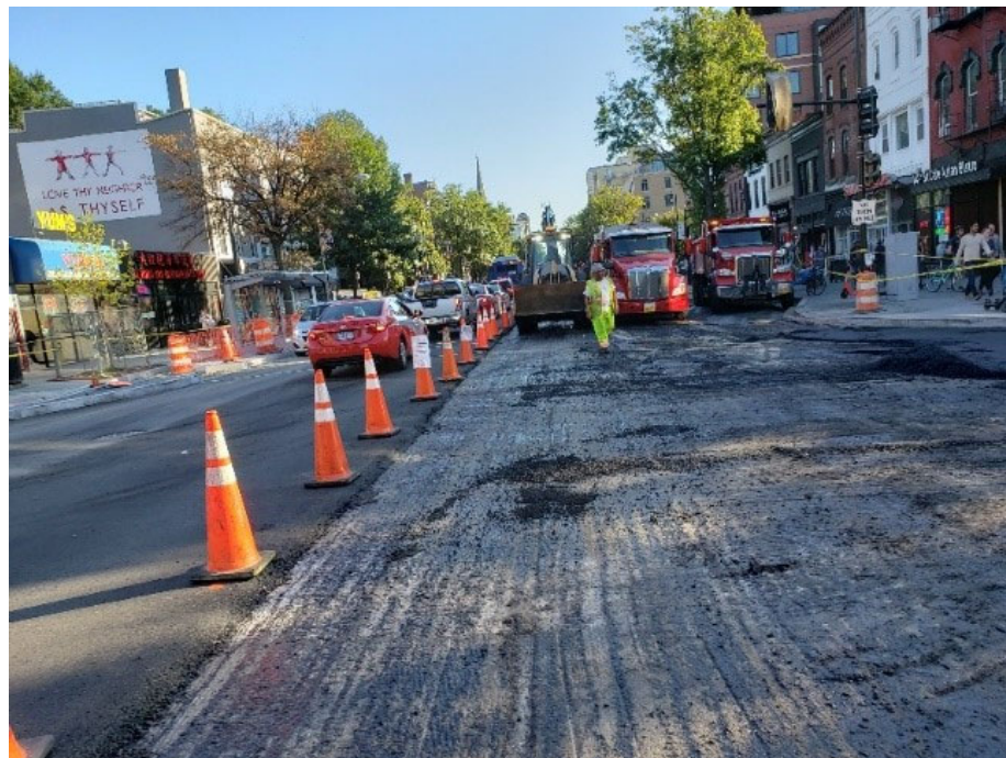
FMCC Asphalt Division placed 350 Ton of 12.5MM Surface Asphalt on Friday, 10-11-2019; P St. to R.I Ave & 14th St.
