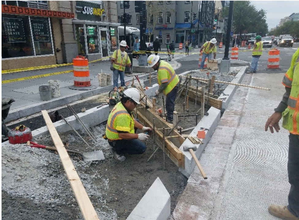
Interceptor drain channel formed by FMCC at NEC of U St
