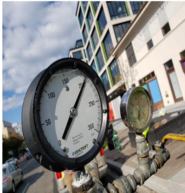
OMNI, Inc. crew along with DC Water Inspector conducted Water Pressure Test for the new Water Main on Wed. 10-9-2019, at Corner of R St. & 14th St. NW.
