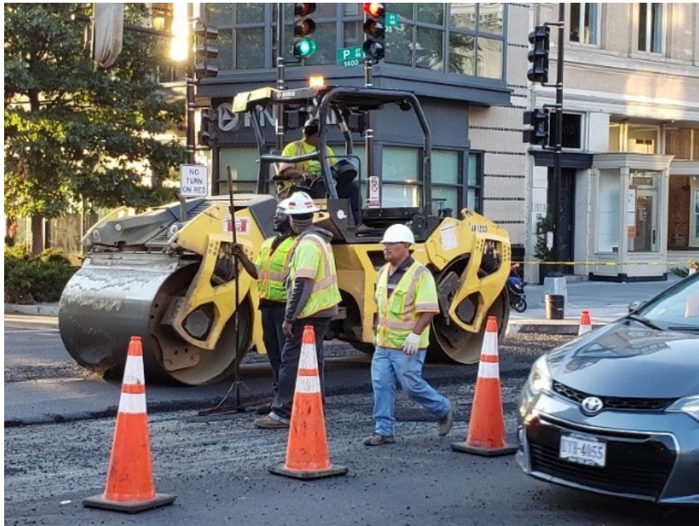
FMCC utilized Flaggers and Spotters to direct Peds, Bike and Vehicle Traffic during Paving Operation at 14th St. from P St. to R.I. Ave. NW.
