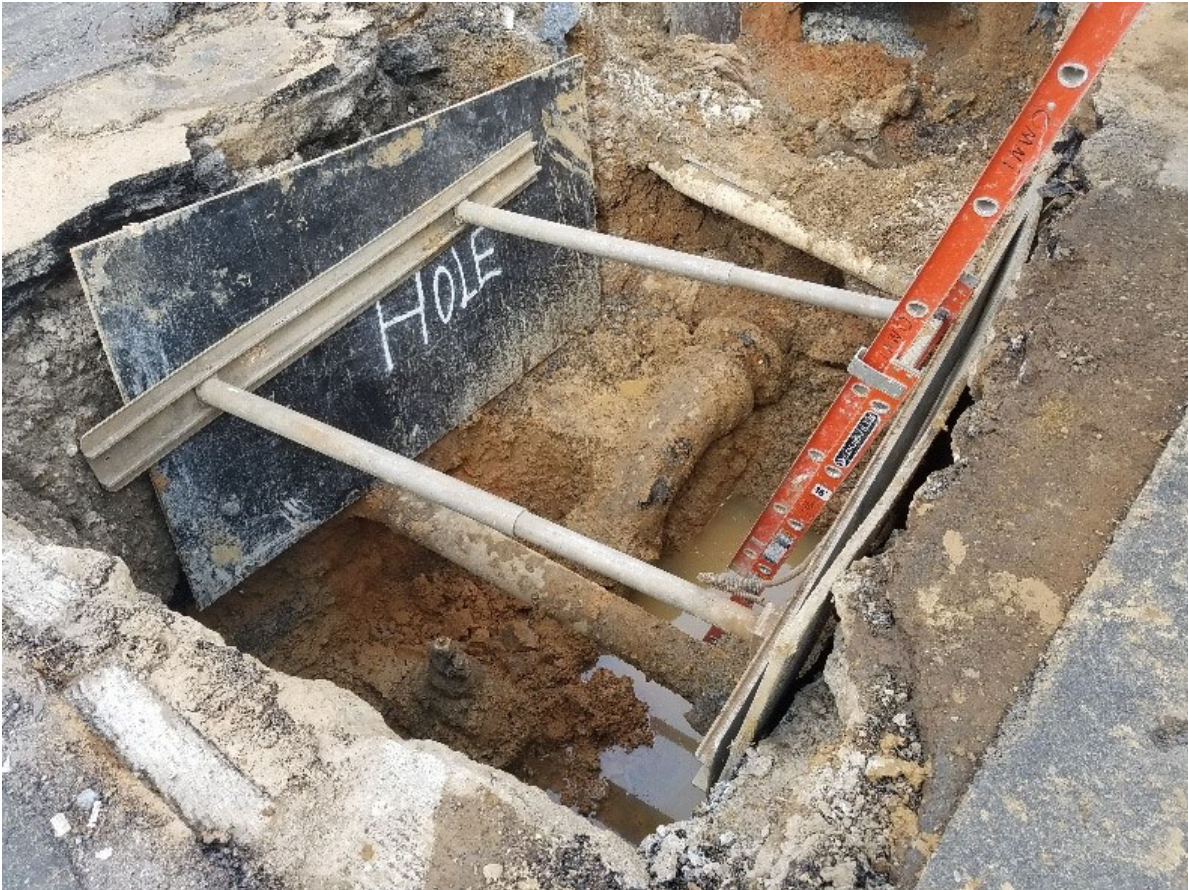
Omni working at NEC of 14 th & R St preparing for water main tie-in.
