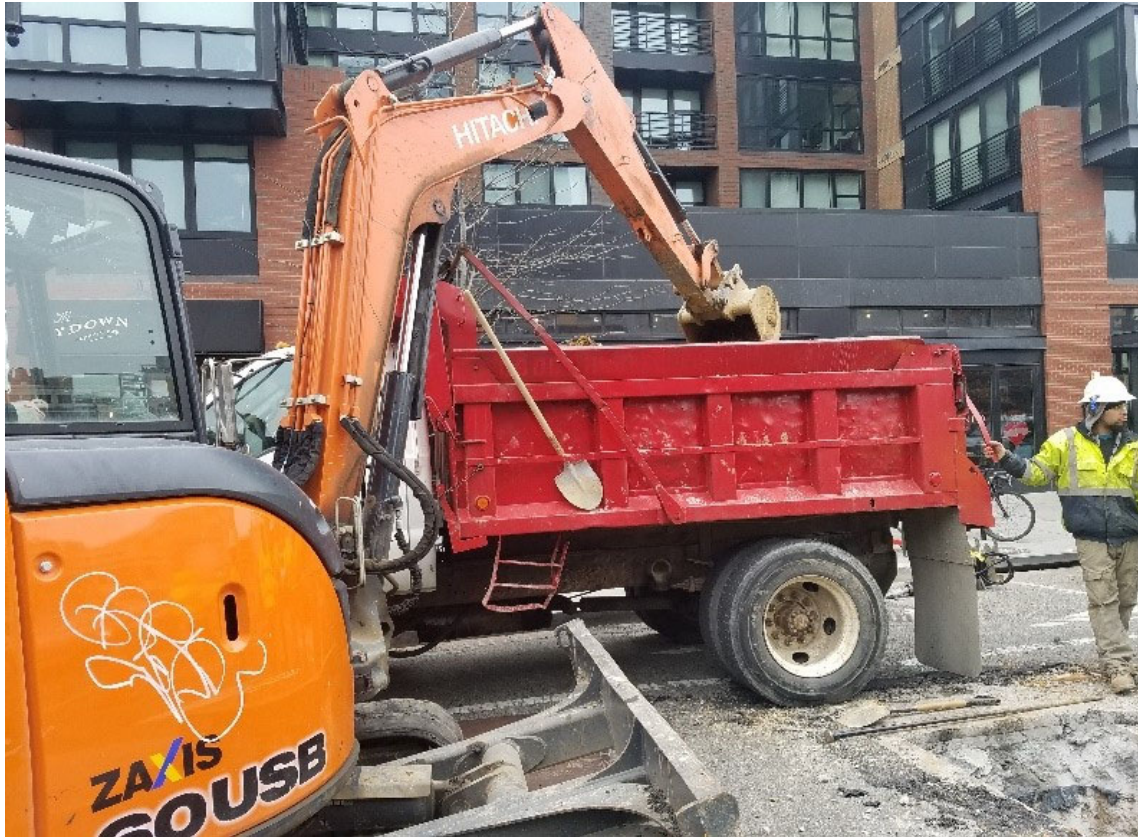
Omni excavating trench for future tie-in at fire hydrant near Wallach St
