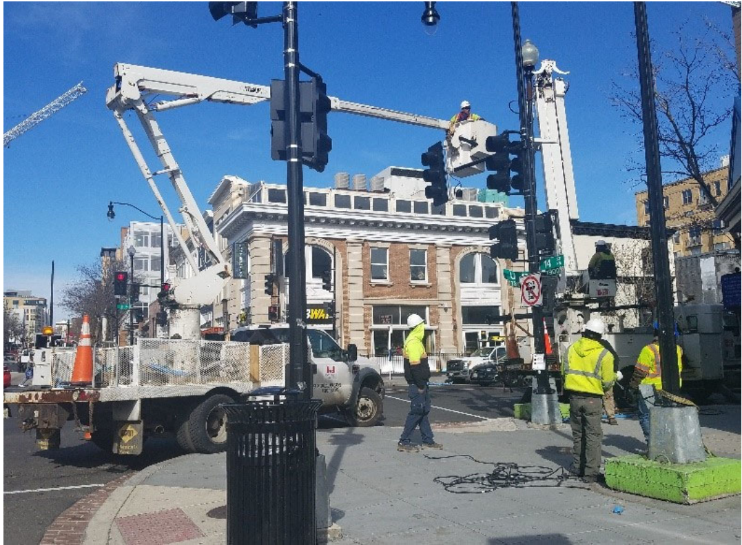
FMCC electrical crew at SEC of 14 th & U St installing APS Unit w/ custom messaging at L96.
