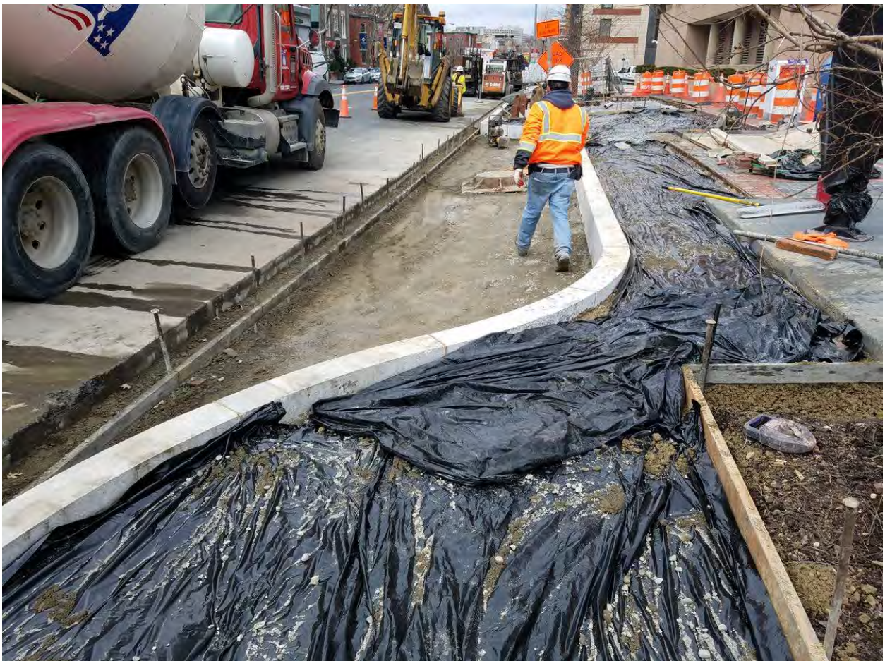
Installation of Bump in and PCC Sidewalk at 14 th and U Street
