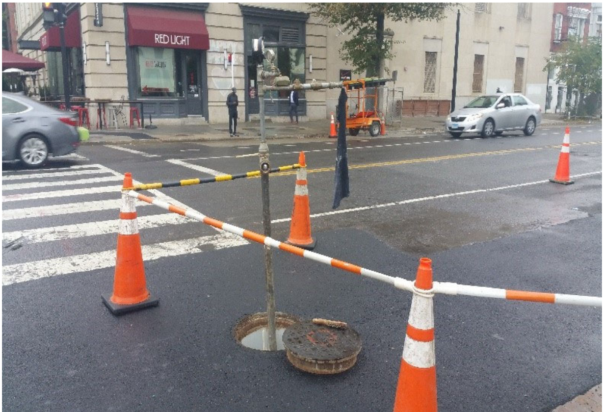
Blow-off valve at northbound 14th & R St
