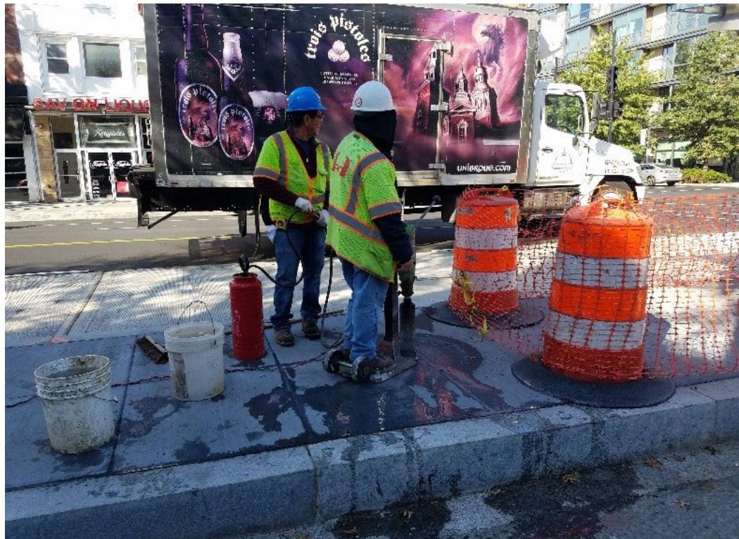
Location near SEC of 14th & T St where bus pad was removed for new directional bus island.
