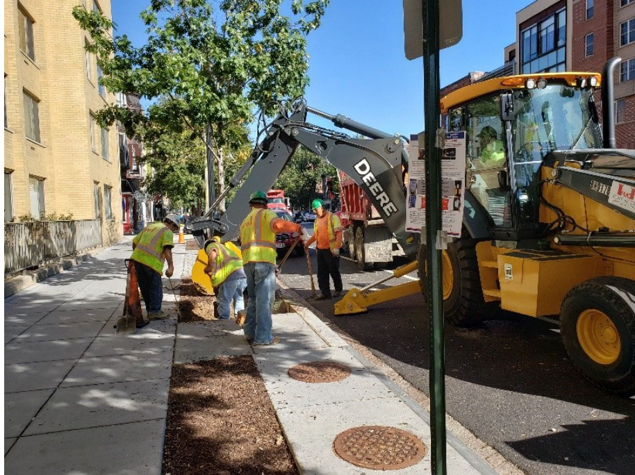
FMCC crew continued excavation Tree Box Planters for preparation for Cooper Landscaping, Inc. to place Str. Soil and Top Soil for Tree Planters. Monday, 10-14-2019 Near N St. & 14th St. Intersection.
