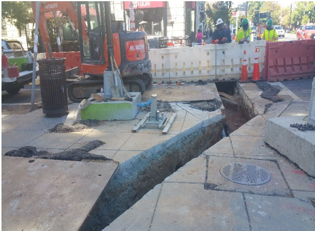
Steel plating at SWC of 14th & R St removed for concrete placement
