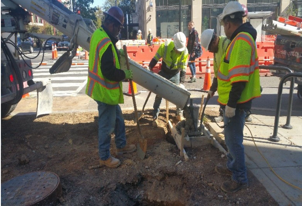
Class B concrete placed at L57 at SWC of 14th & R St
