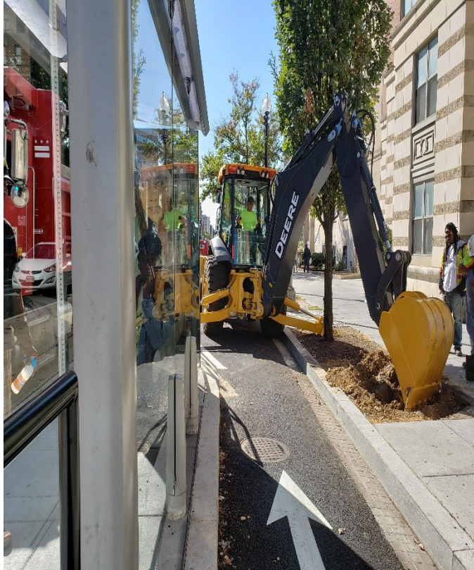
FMCC crew excavated for Planters near Bus Island Shelter at 1200 Block of 14th St. NW & N St. Intersection at SB.
