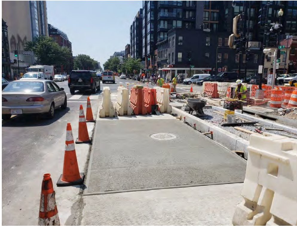
Finished 4500 psi concrete surface of bus pad & adjusted PEPCO man hole vault
