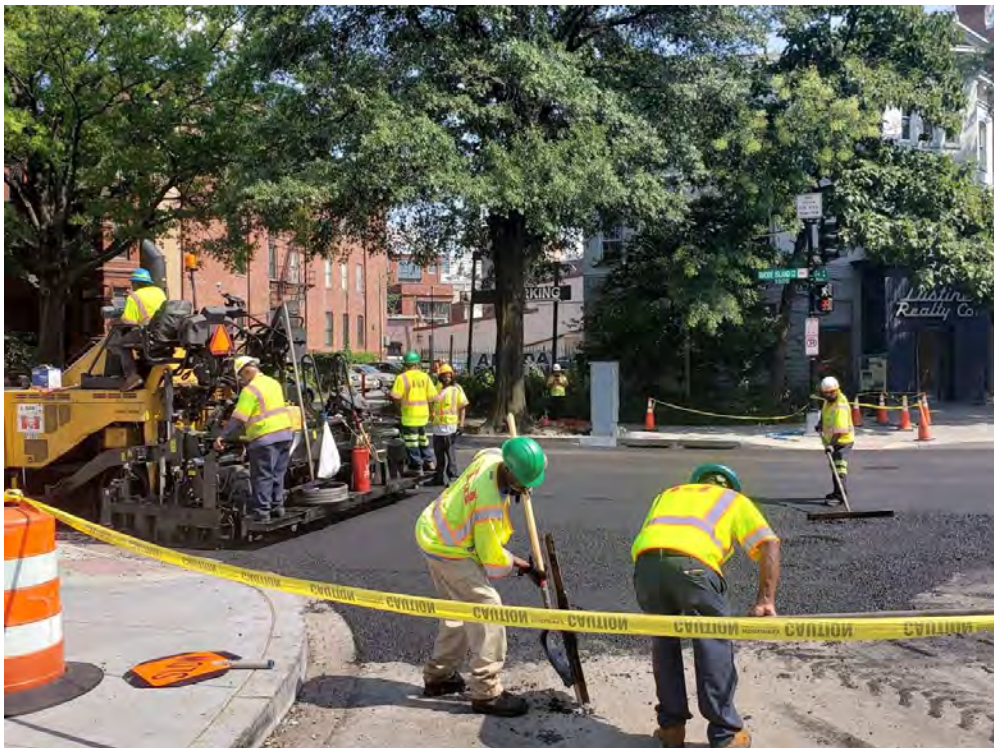
Asphalt paving at the intersection of 14 th St. NW & Rhode Island Ave.
