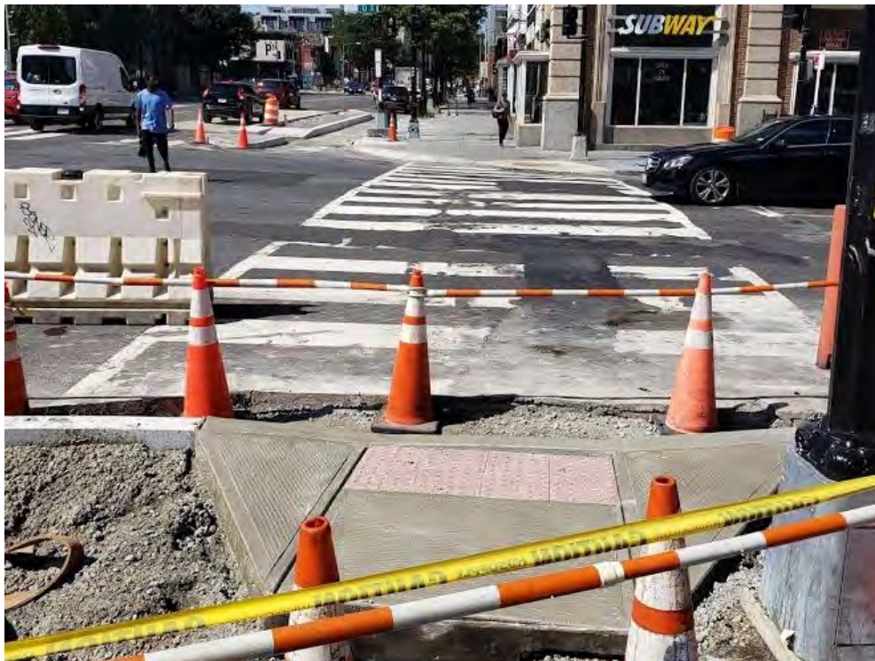
DEN Construction completed ADA ramp at the corner of 14 th St NW & U St.
