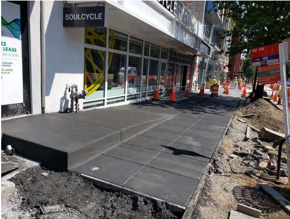
DEN Construction completed sidewalk and ramp at 1900 block of 14 th St. NW
