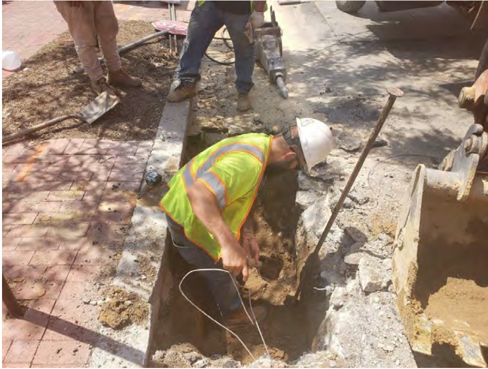
Test pit for underground utilities prior graded inlet install at 14 th NW & T St.
