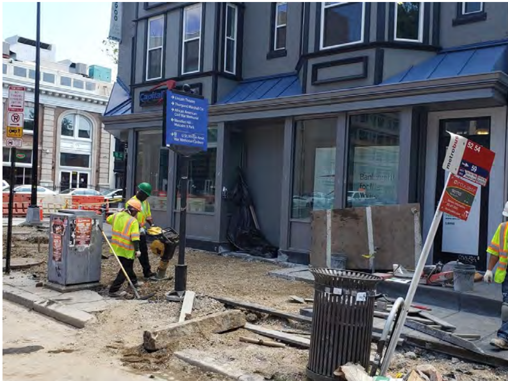
Excavation & compaction of GAB prior to sidewalk concrete install at 1925 14 th St. NW
