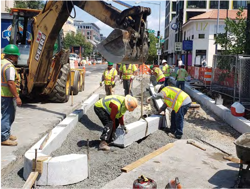
FMCC install bus island with dry concrete mix at 14 th St. NW & R St.
