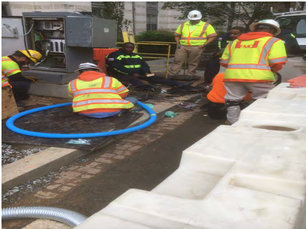
PEPCO, DDOT, and FMCC working on the Transfer of the Traffic Control Cabinet at N Street
