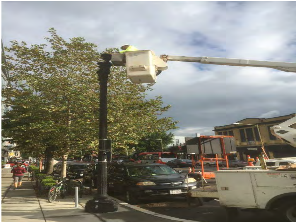
Installing the 100-watt LED and Globes on the Twin 20 Street Light Poles
