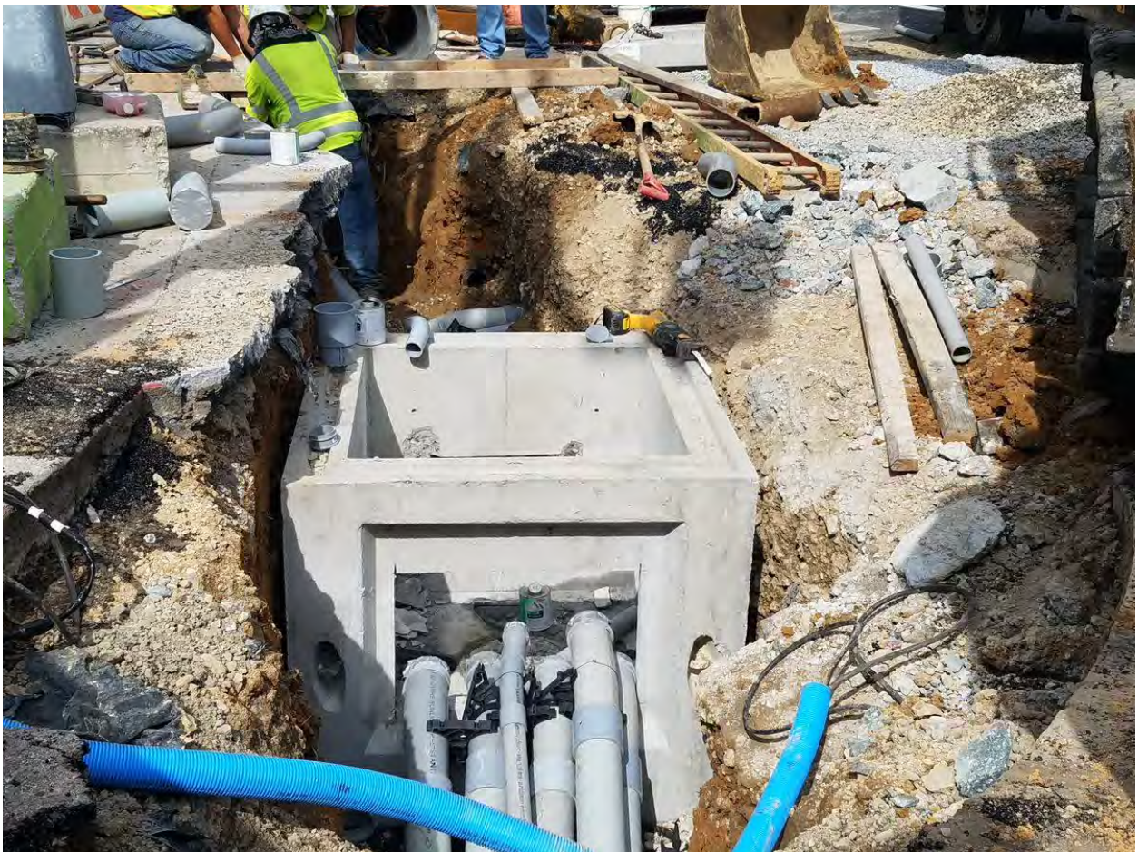
Installation of Manhole and Electrical Conduit at the NW Corner of 14th and P Street
