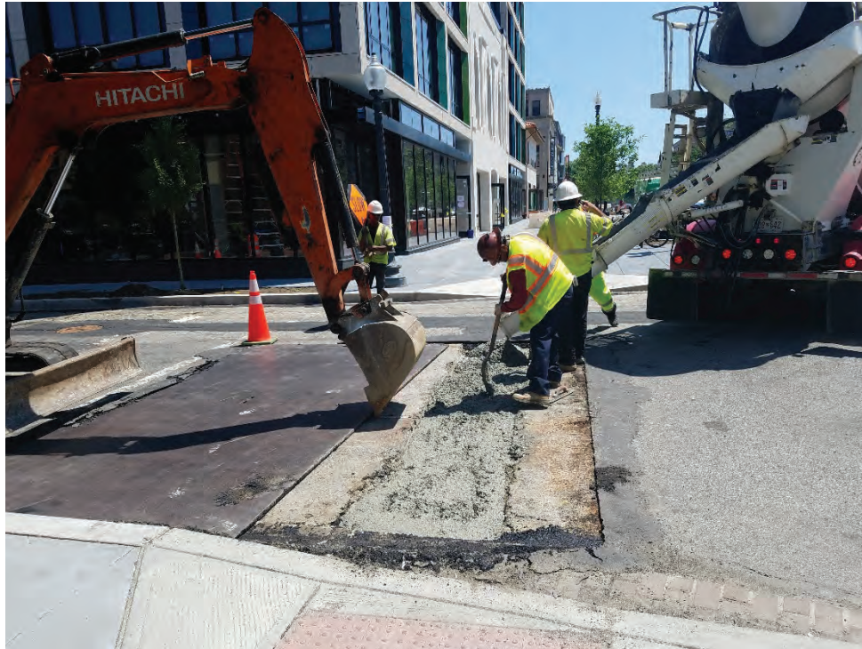
PCC Base placed at 14 th & Riggs St atop encased PVC conduit run.
